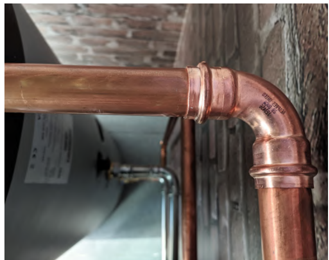
Image 16 - aesPRES UNIKO - Installation de chauffage
